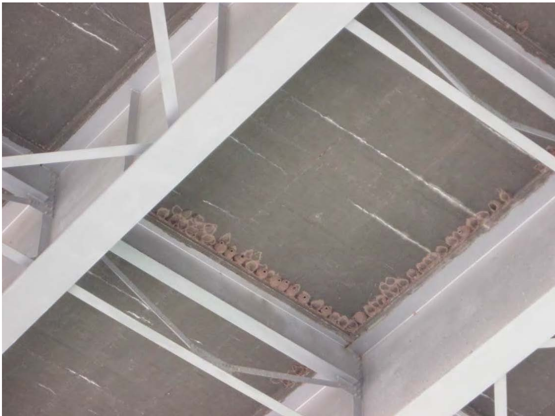
Photo 8. Cliff swallow nests attached to the underside of Bridge No. 1.
