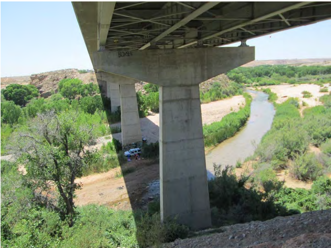
Photo 2. East side of I-15 at Bridge No. 1 and Virgin River looking west.
