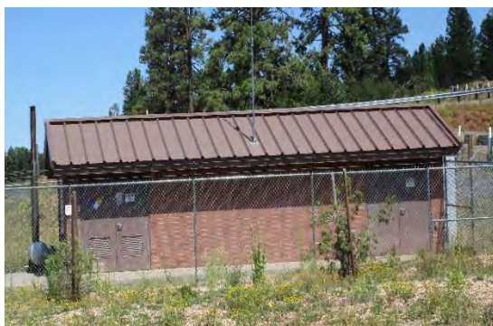
Airfield Lighting Electrical Vault Source: Coffman Associates
