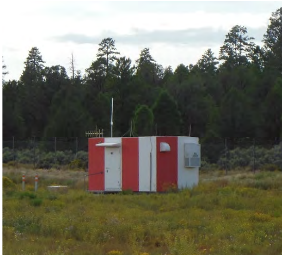
Localizer Equipment Shelter
