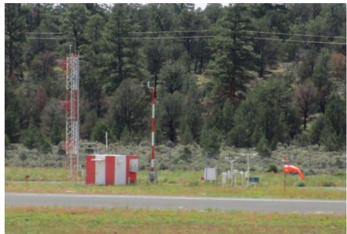
Instrument Landing System (ILS) Glideslope Antenna and AWOS-III Equipment
