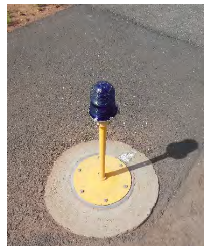
Medium Intensity Taxiway Light (MITL)
