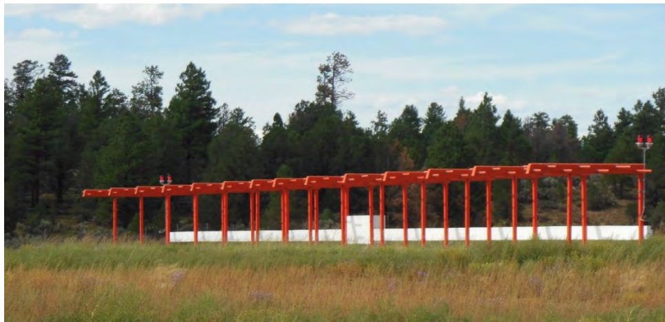
Instrument Landing System (ILS) Localizer Antenna Array
