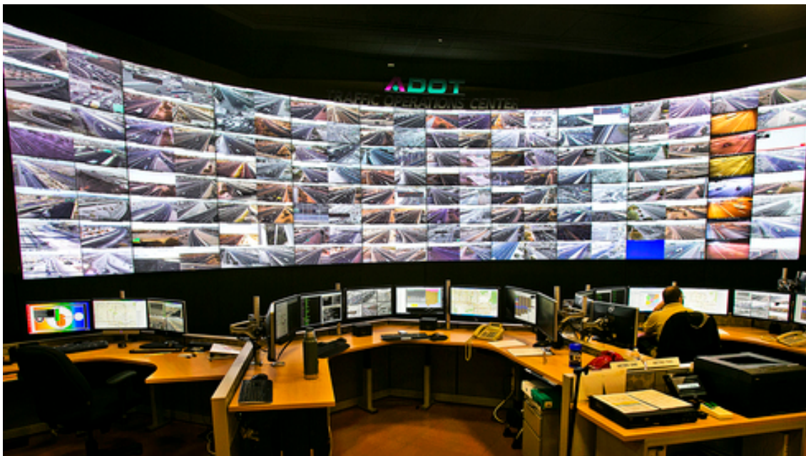
Figure 3 – ADOT TOC Operations Room
