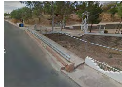
c) The sidewalk steps up on the bridge across the Ephraim Canyon Wash on Western Ave
