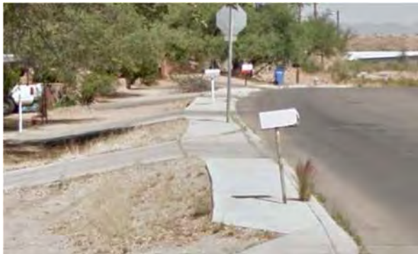
a) Mailboxes may obstruct the sidewalk towards the western end of Target Range Rd.
