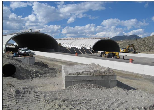
Figure 3- 1. Precast concrete arch wildlife overpass being constructed on I-80 in Nevada as a stand-alone drop-in structure project.
