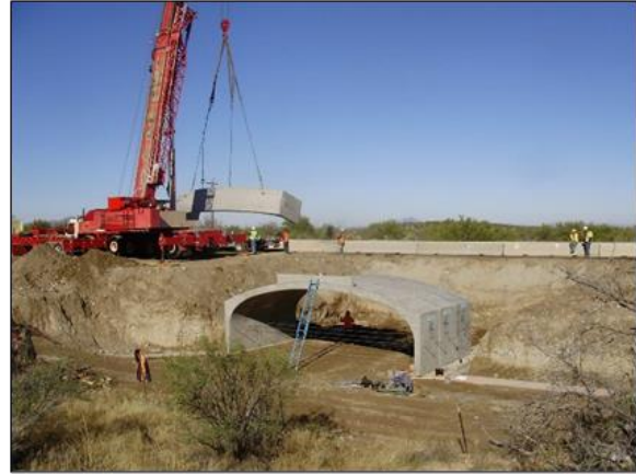
Figure 3- 53. Installation of a drop-in precast arch wildlife underpass along SR 86 with similar dimensions to that recommended for SR 77.
