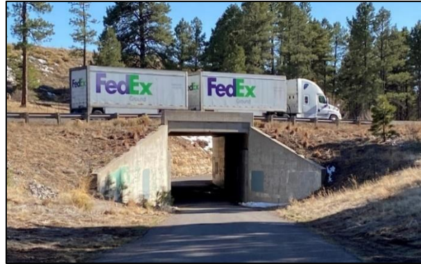
Figure 3- 38. The large access road concrete box culvert under the WB lanes of I-40 located at MP 197.6, looking south.
