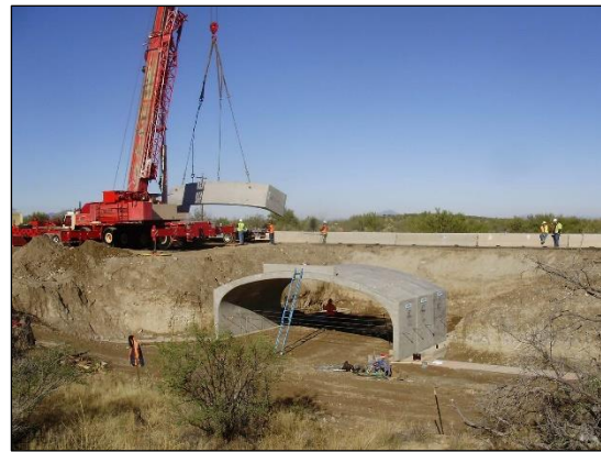
Figure 2- 19. Installation of the first half of the drop-in SR 86 Kitt Peak arch underpass in 2011.
