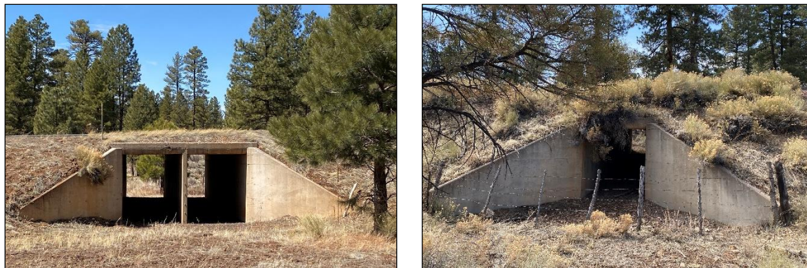
Figure 3- 23. Existing CBC along SR 64 Hotspot #2, one a 2-barrel structure (MP 232.5; left) and the other a single-barrel CBC like all other structures (right), with fencing at the mouth that limits wildlife access to and through the already marginal structure.
