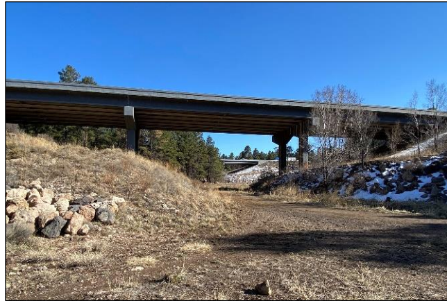
Figure 3- 32. The Rio de Flag bridges on I-40 (MP 197.5) under which the Rio de Flag flows.
