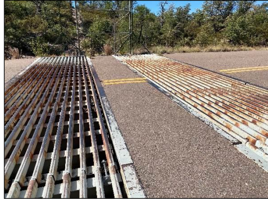
Figure 3- 94. Improperly designed/ installed double-wide cattle guards on the SR 260 Little Green Valley Section that may be contributing to WVCs.
