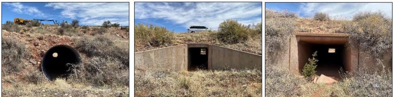
Figure 3- 45. SR 77 Hotspot #4 drainage structures including large, corrugated metal pipe (MP 350.9; left), and CBC at MP 351.74 (center) and MP 353.35 (right). All are marginal for wildlife passage (see Table 3-14 for dimensions).
